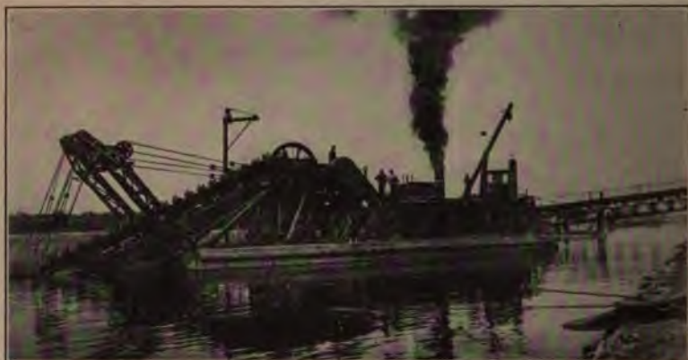
View of Excavating End of Steel Pontoon Dredge Operating on New York State Barge Canal.
